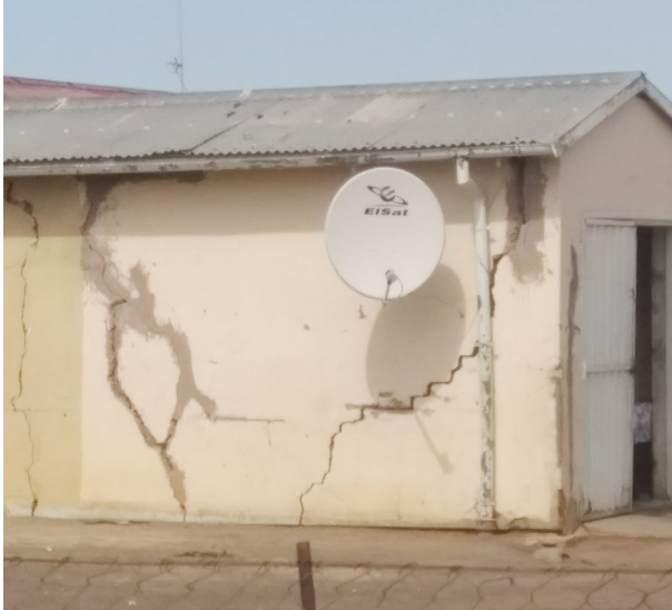
Figure 112: A house in Mariental with wall cracks, a phenomenon common in the town and affecting the property market in the area
