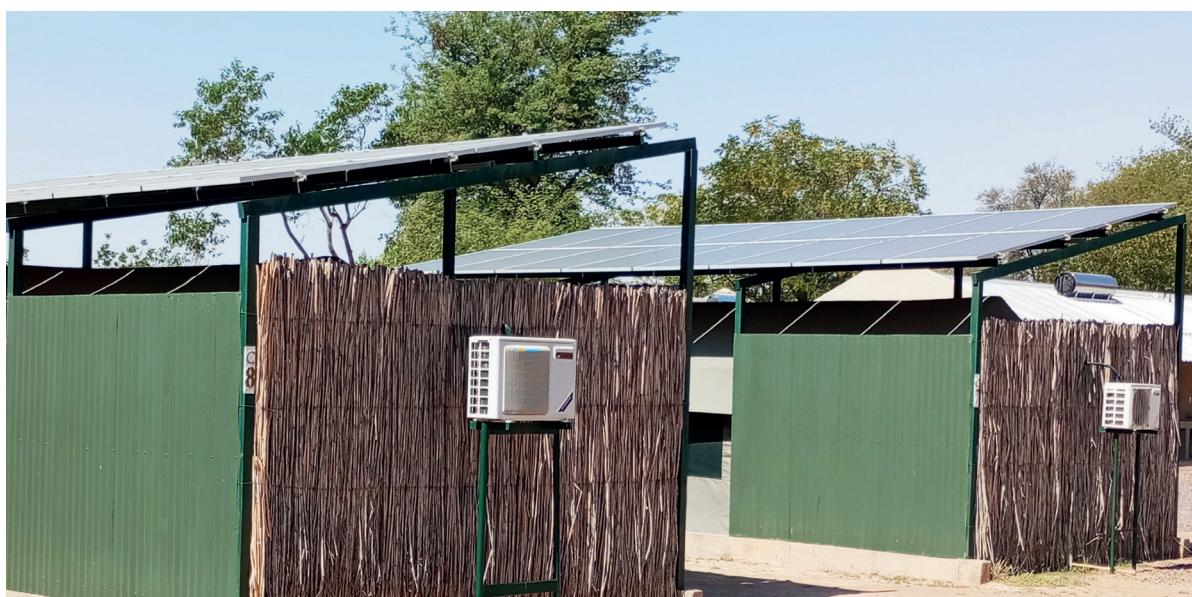
Figure 46: An example of the air condition system powered by solar panels on a partially thatched structure in southern Namibia
