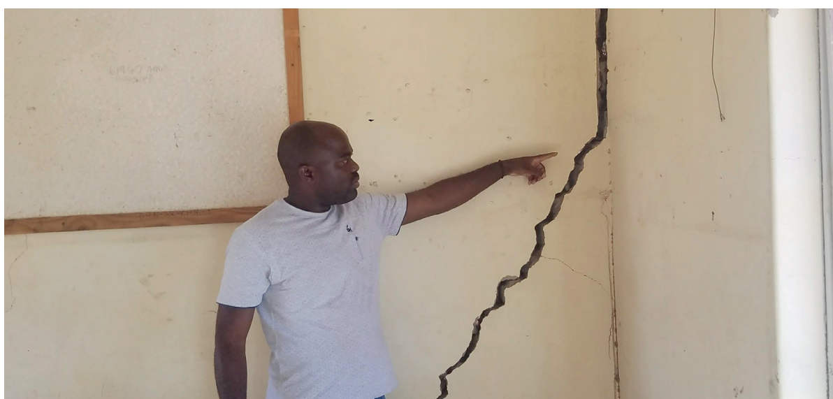
Figure 66: The office of the //Gaoio Daman Traditional Authority in Anker, Kunene Region, damaged by earthquake
